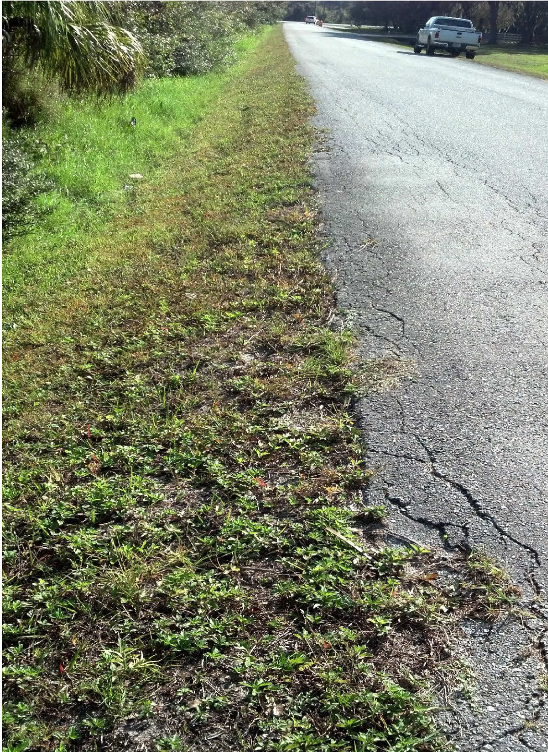
Damage to pavement on the roadway edge due in part to a lack of roadway shoulder to hold the base and pavement in place.
