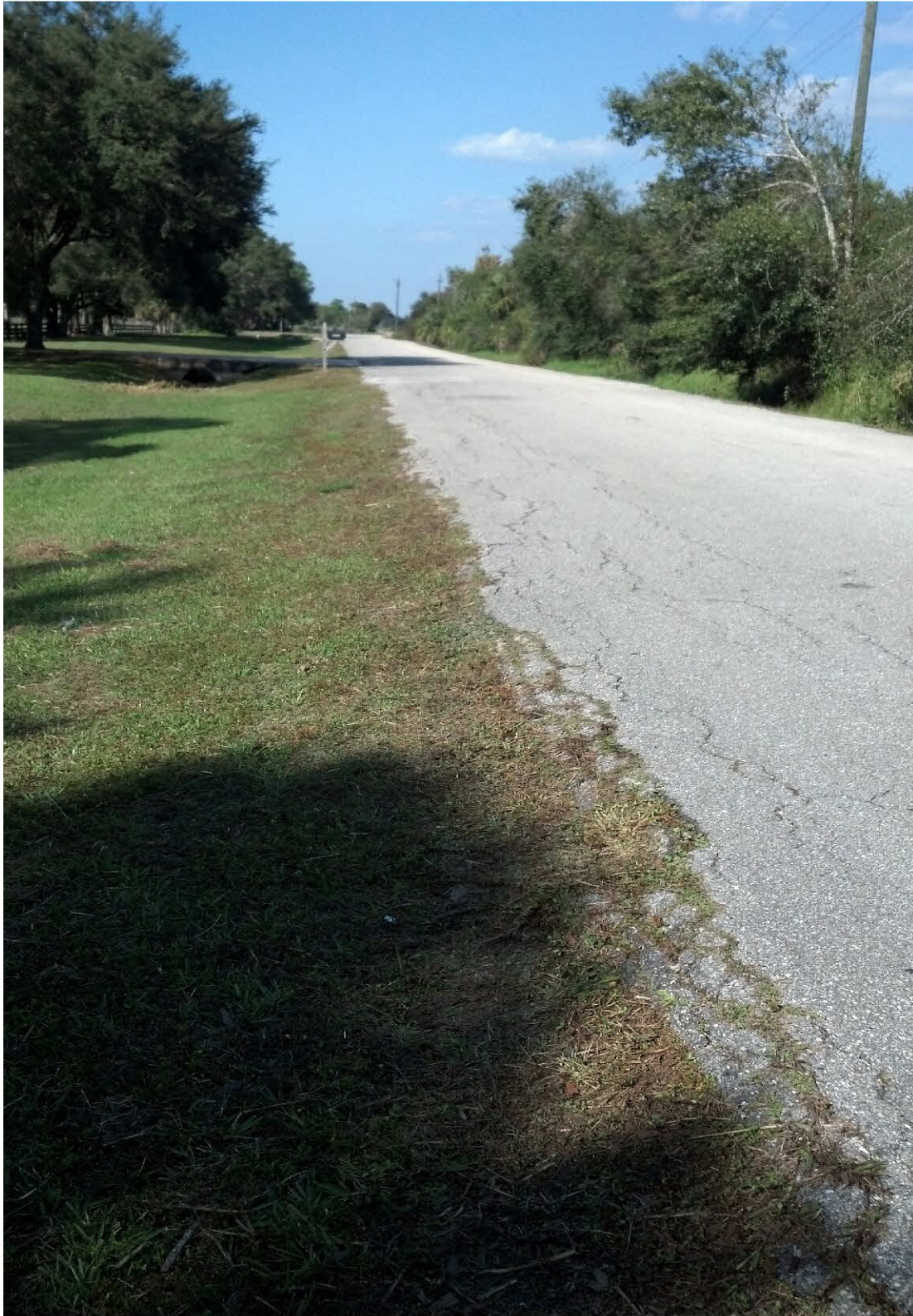
Damage to pavement on the roadway edge due in part to a lack of roadway shoulder to hold the base and pavement in place.
