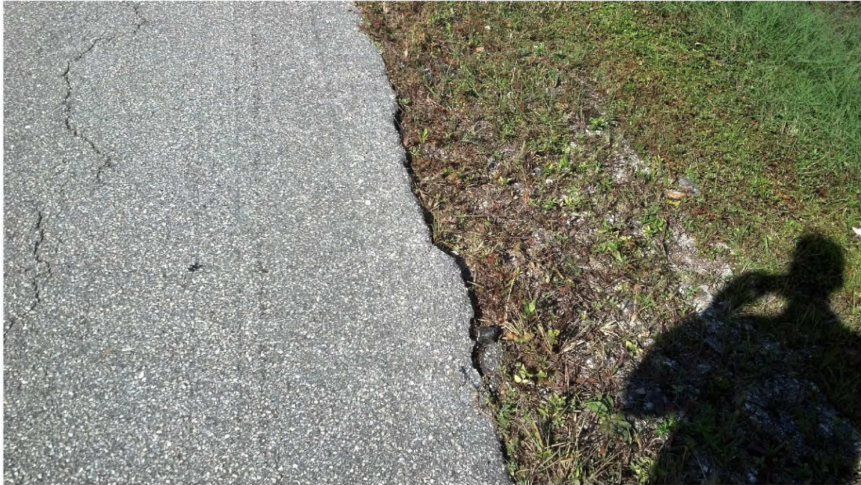
Roadway edge damage and subsidence due to lack of should to hold roadway base.
