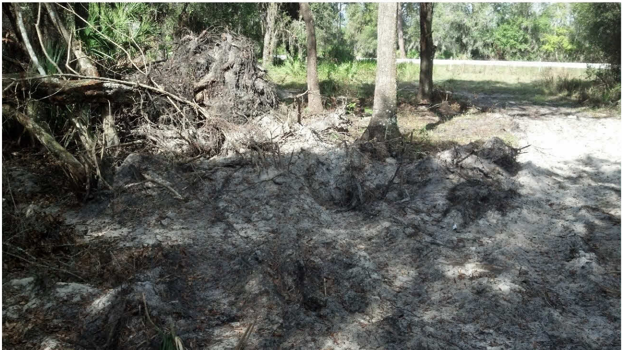
Additional views of the clearing and filling of the channel of Cowpen Slough south of Fruitville road. Note the existing ditch of the channel in the left hand side of the photo.
