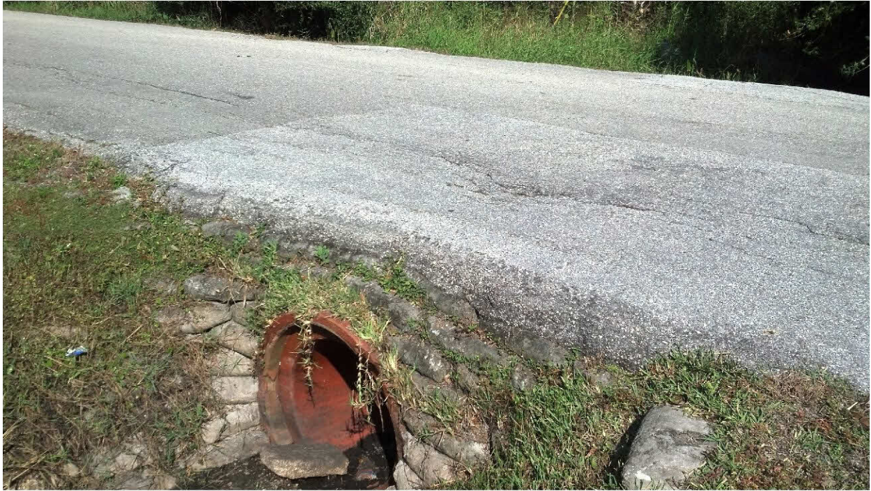
Culvert end without mitered end section extending out past the clear zone for traffic. This condition creates a hazard to vehicles that may drift off of the road wan into the ditch.
