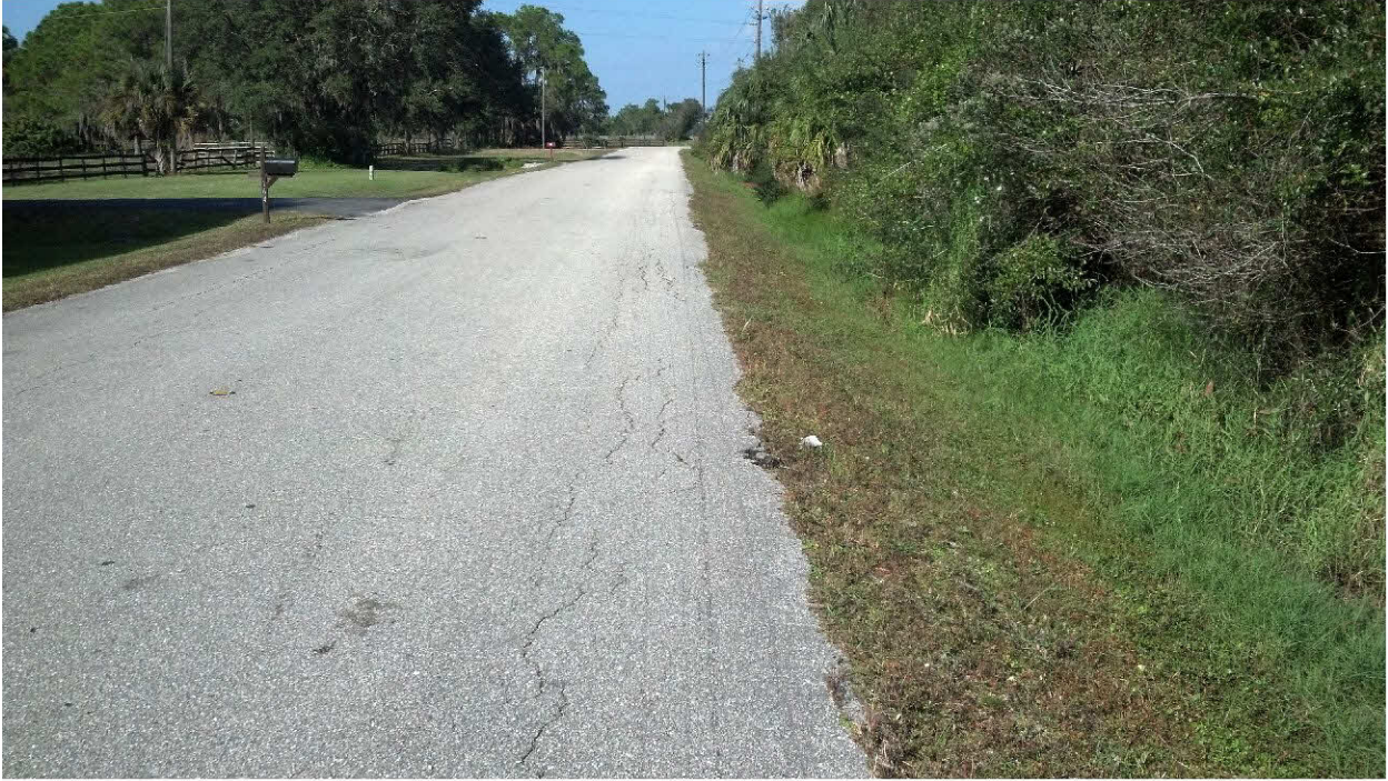
Cowpen Lane cross view showing no or minimal shoulder on east side of road.
