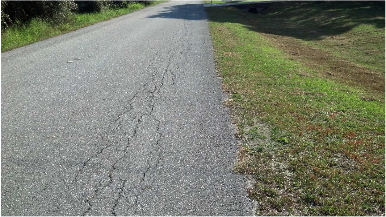
Rutting visible on outside wheel lane of roadway.
