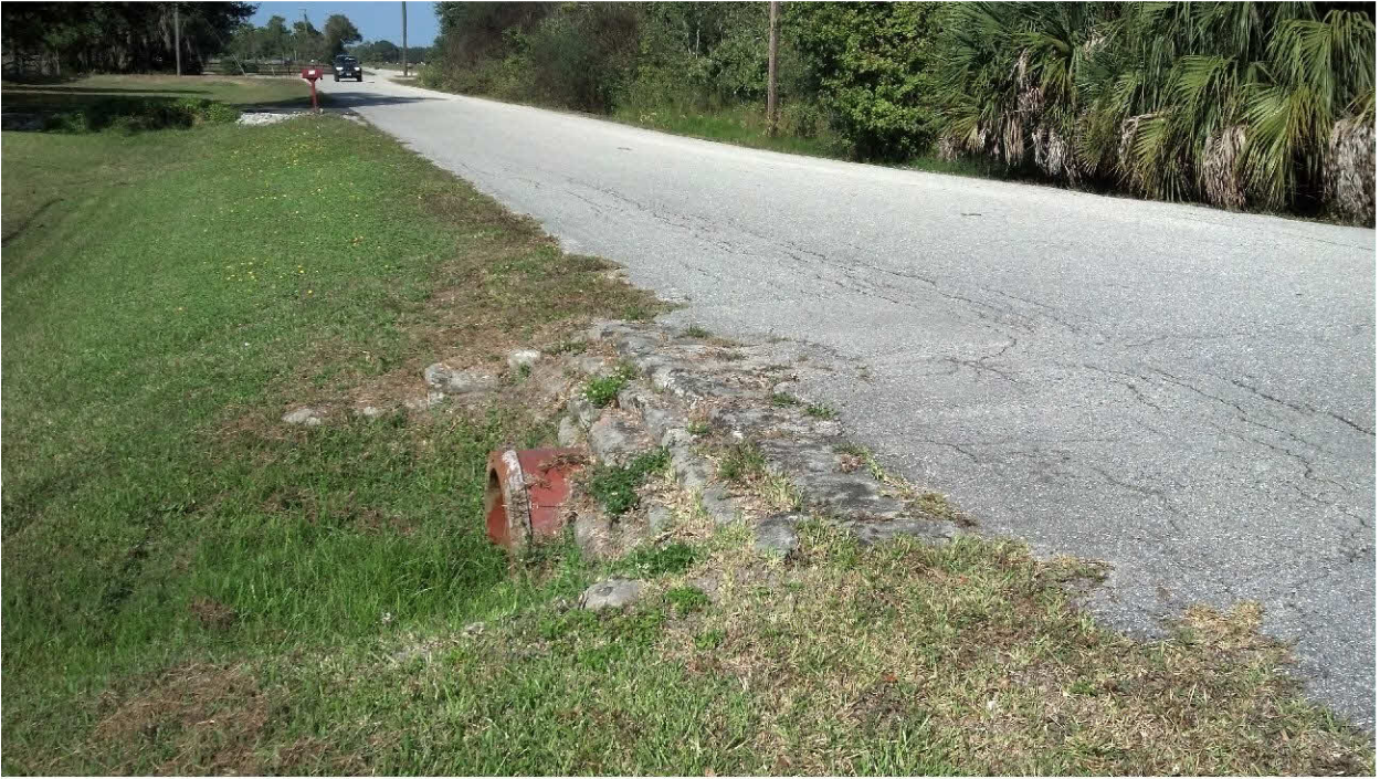
Culvert end without mitered end section extending out past the clear zone for traffic. This condition creates a hazard to vehicles that may drift off of the road wan into the ditch.
