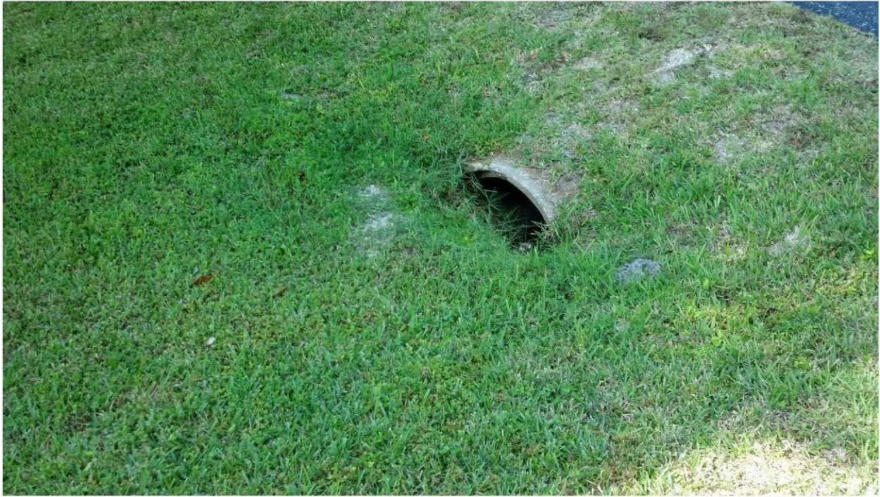
Partially clogged culvert under driveway on west side of Cowpen Lane.
